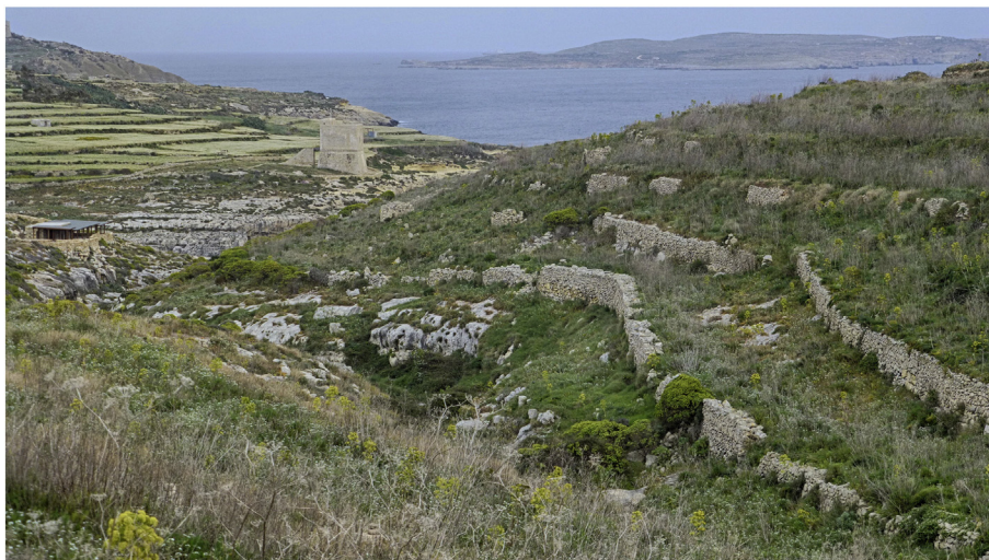
Fig. 22. Agricultural terraces on Gozo (Malta) (pm 10-1). The collapse of the terrace walls on the right slope released formerly stored sediments. The hill on the left side shows still intact soils with a thickness of up to 1 m (picture taken on 02.04.2013 by the author).
