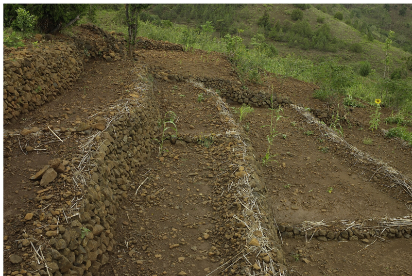
Fig. 11. Newly constructed 'Living Terrace' near Konso (pm 3-3) in the highlands of southern Ethiopia (picture taken on 30.12.2009, courtesy of H.-R. Bork).
