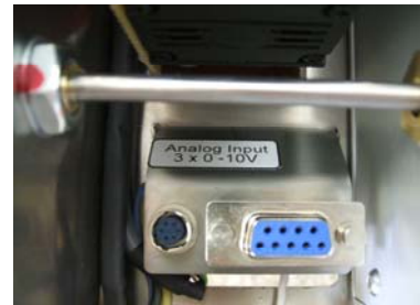
Figure 11: RS-232 connection at the docking-station
